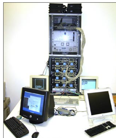
Figure 3. Hardware for the Arch-OS control system at the Portland Square Cybrid Building
